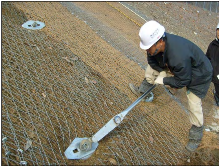
Tightening of the nut to the required torque using a torque wrench.
