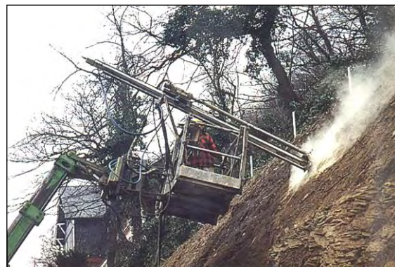
Example: Depending on terrain conditions, drilling work can also be carried out from a small crane platform or lifting platform.
